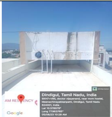
Water Tank in New Building – 6
