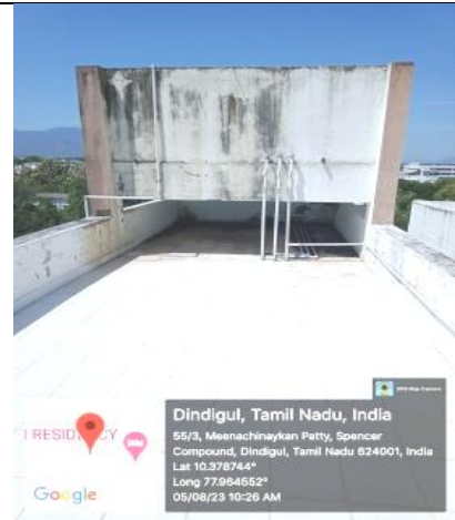
Water Tank in New Building – 5
