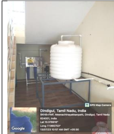
Drinking water Tank – 3
